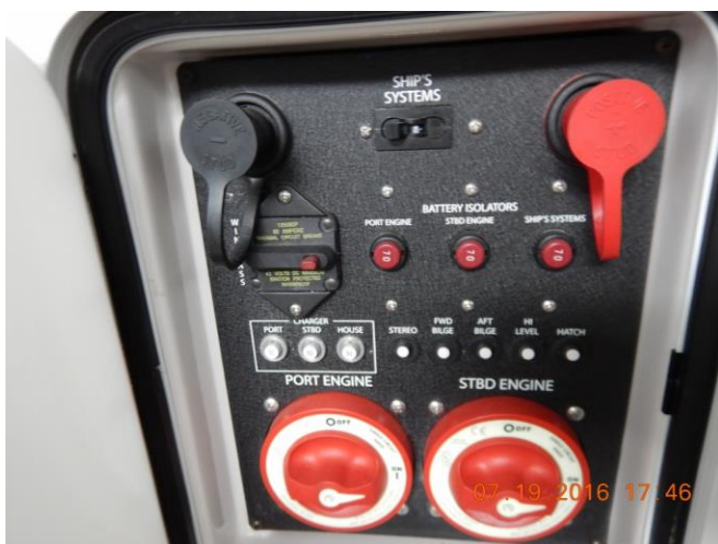
Figure 32 - DC Control Panel in Cockpit
