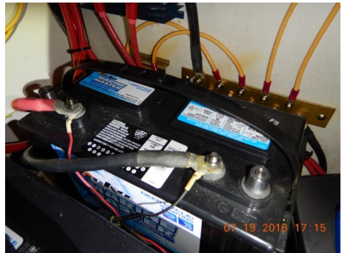
Figure 31 - Starboard Engine battery
