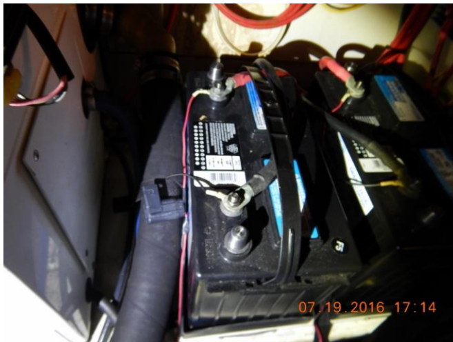
Figure 30 - Port Engine battery
