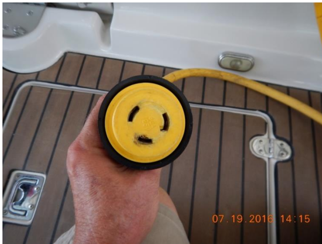
Figure 27 - Air Cond Shore Power Cable connector excessive heat damage
